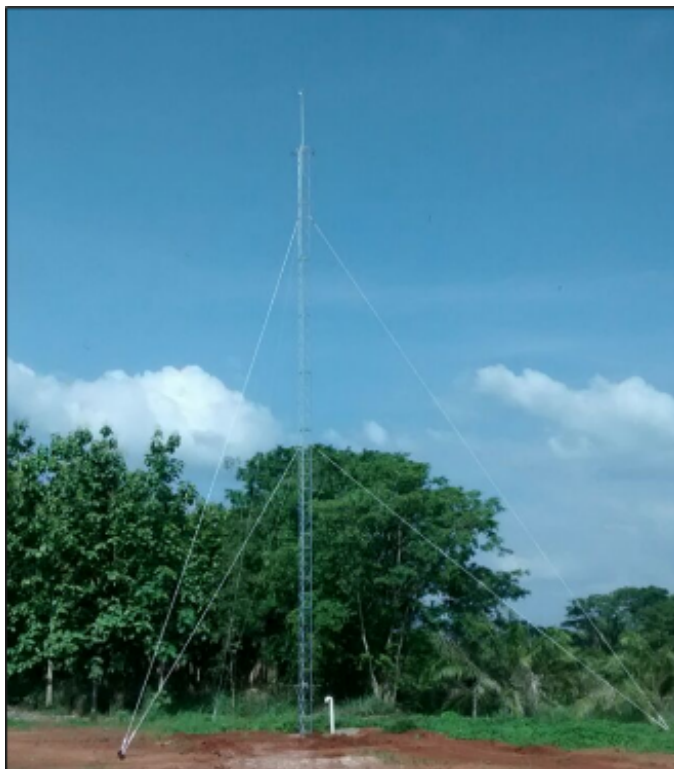
Figure 21: CADI transmission antenna installed at Araguatins observation station.
